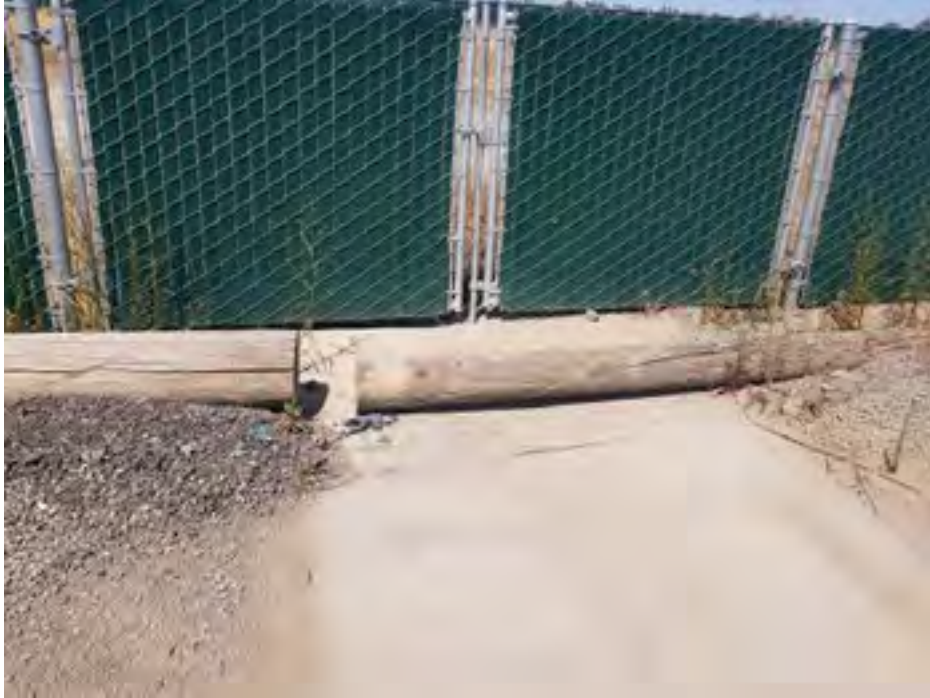
Figure 2.2-11 Sangha Trucking Yard Drainage Infrastructure
